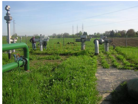
Cleaning station Topolovac
