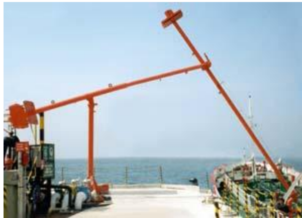
Figure 3 Loading arm being used to transfer fuel to a waiting barge.
