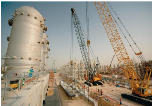
Figure 33. FT reactors at Shell's Gas-to-Liquids plant Pearl GtL in Qatar (production \approx 7 \times 10^9 litres/year).
